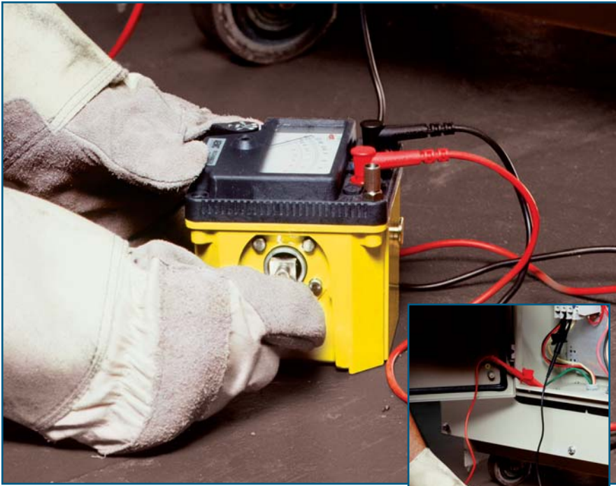
Model 1250N performing a hand-cranked 1000V test on a generator.
